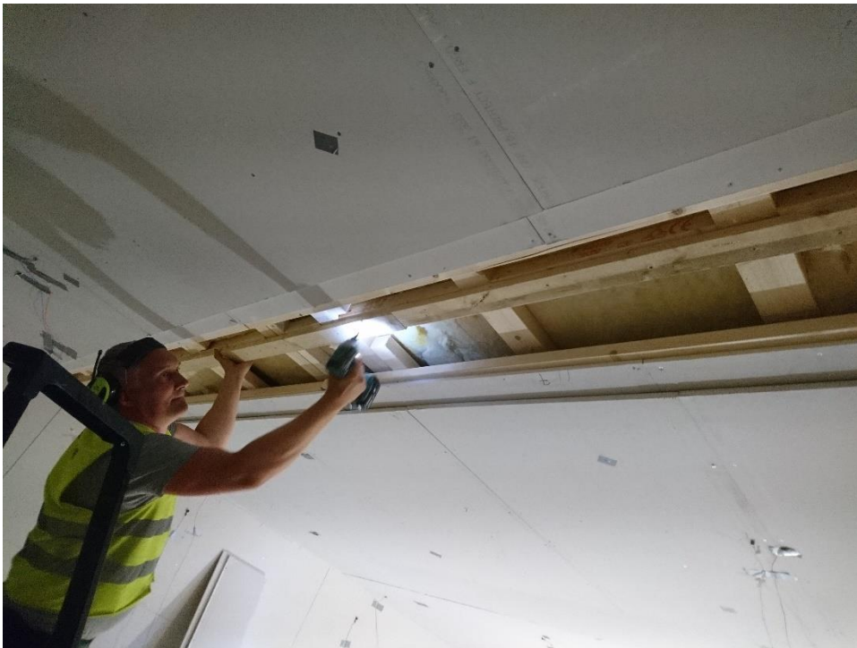
Figure 10. Test setup version 5, Screwed and glued lath to create composite action of nogging rows. Second gypsum layers added before measurements.
