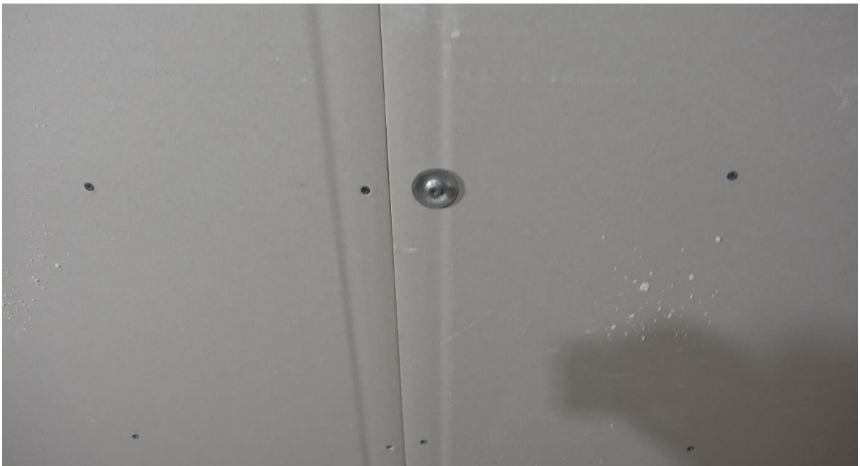
Figure 8. Test setup version 2, fastening the gypsum boards against the ceiling joists with screws and washer to take away the suspended ceiling effect.
