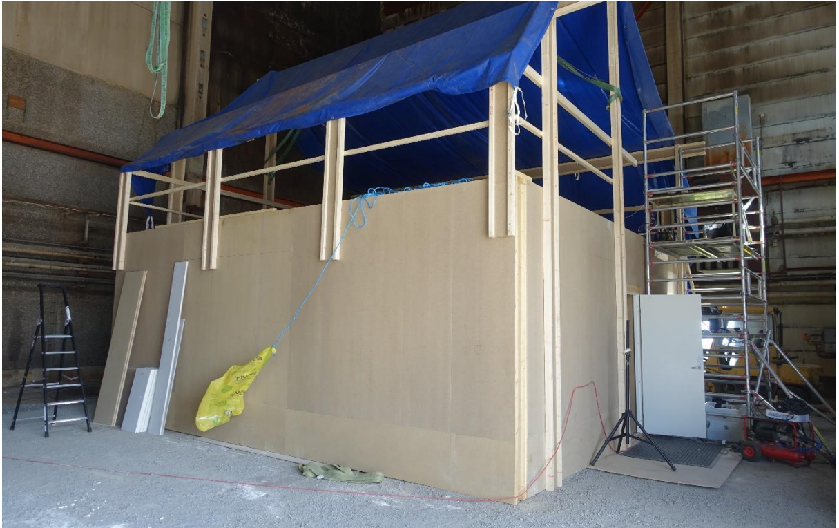
Figure 5. The test houses at the measurements with the scaffolding as a platform for the measurement system. The test house walls are standing on gravel. The test house is located within a large industrial building at Masonite Beams in Rundvik. The scaffolding is not connected with the test house structure.
