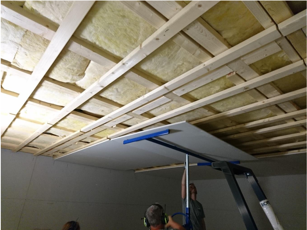
Figure 7. Mounting of the first layers of gypsum boards, test setup version 1. The laths which the gypsum boards are fastened to are suspended (you may note a small distance between the laths and the structural beams above).
